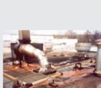
BEFORE: A traditional exhaust with an inline fan leaves the roof covered in extremely messy grease and shortens the fan life.
